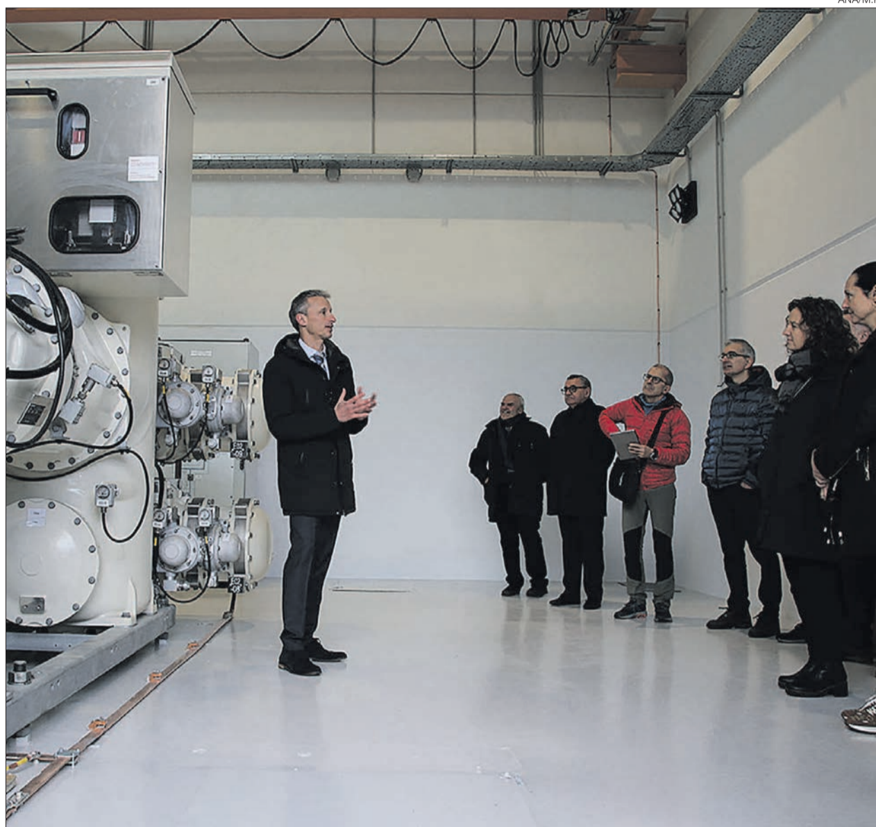
► FEDA's Director of Engineering, Marc Calvet, during the visit to the new facilities.
