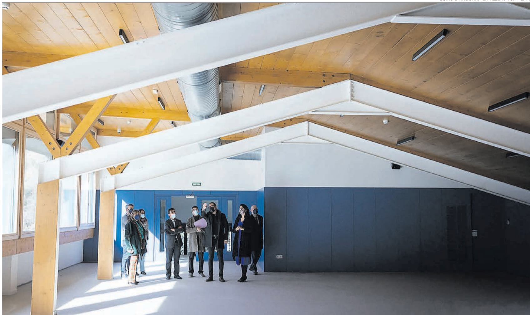
►► The authorities are visiting the progress of the CREI adaptation works, in the last month of February.
