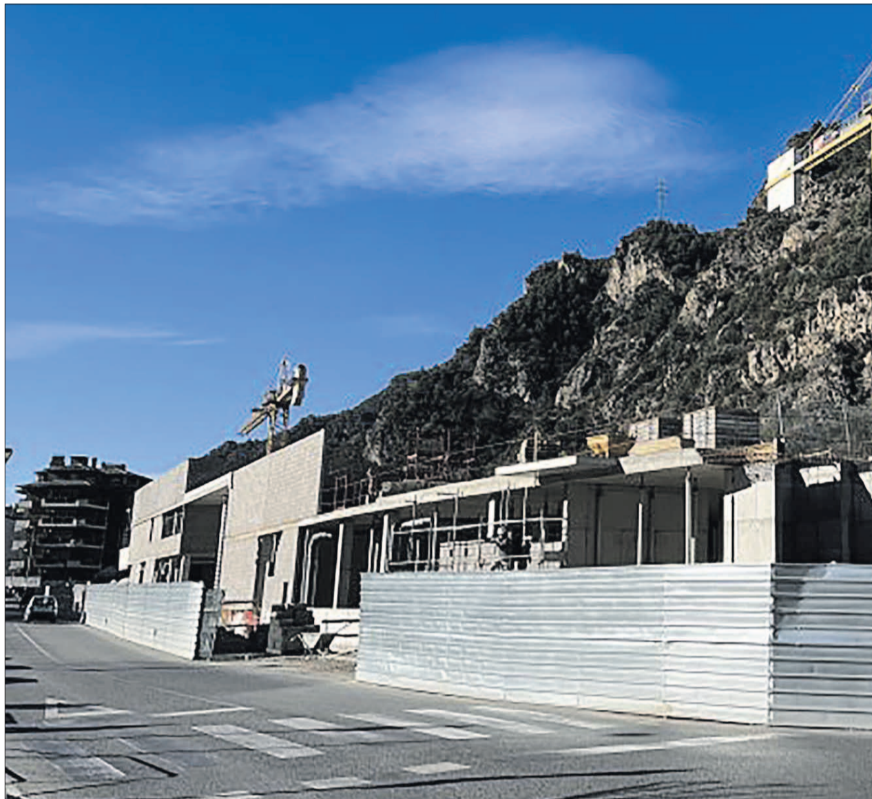
► Construction work on the R15 building in Sant Julià, which will put up to 46 new rental homes on the market.
